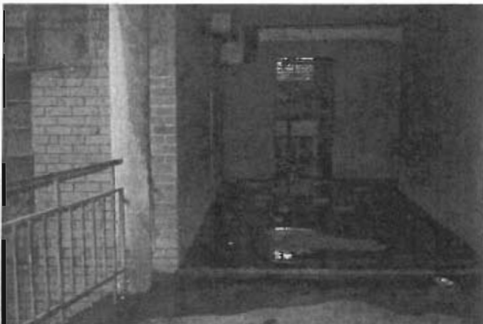
Flooded laundry rooms
