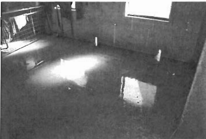
Leaking water from defective water tanker (through ceiling)
