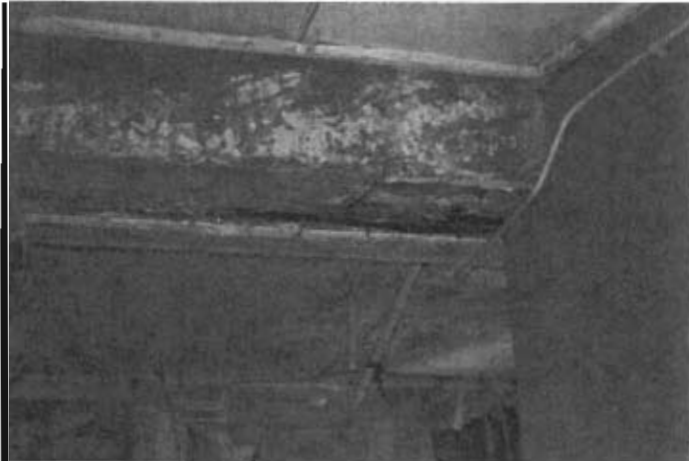
Water damaged ceiling and electricity connection
