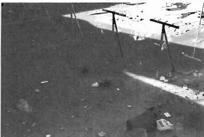
Flooded hostel grounds caused by blocked sewer lines
