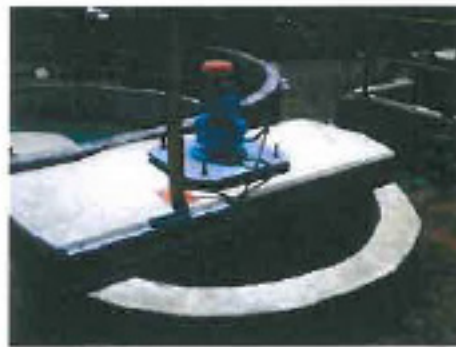
Rapid mixing Chamber
