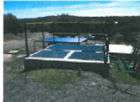
Water dividing Chamber
