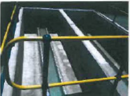
Filters (mat of sand and nozzles)
